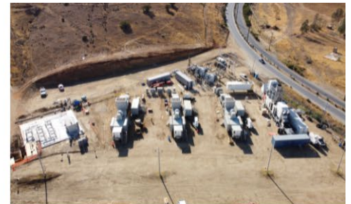
4 turbines operating at Herradura site in Tecate, MX
