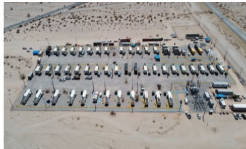
4 turbines and 44 engines operating at Libramiento site in Mexicali, MX
